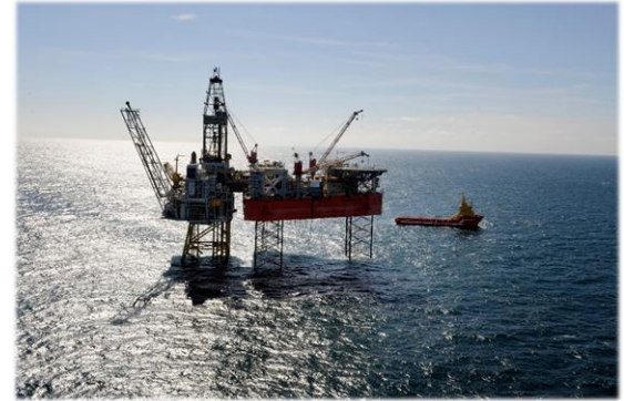
WSP jacked up alongside SNS platform with cantilever skidded out, performing well P&A operations
